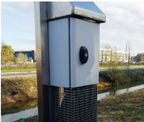
ClareShield WheelPulse measurement unit located trackside
